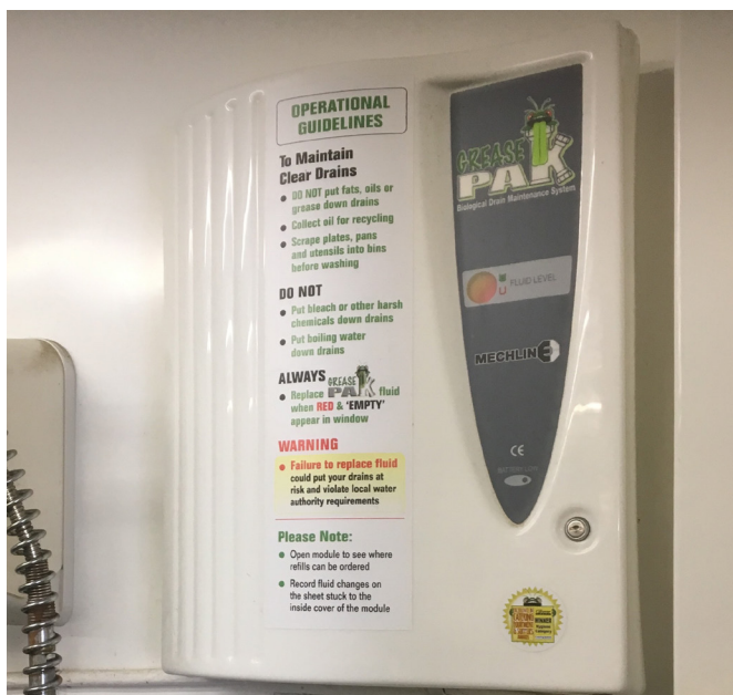
The GreasePak Mark 1 model installed at Alf Turner & Sons, since 2008.
